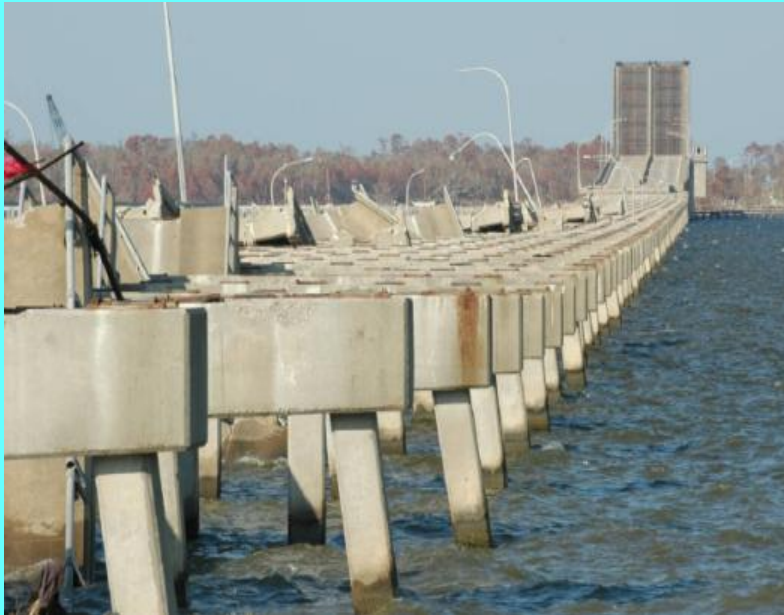
Bridge carrying US-90 damaged during Hurricane Katrina (Douglass et al. 2006)
